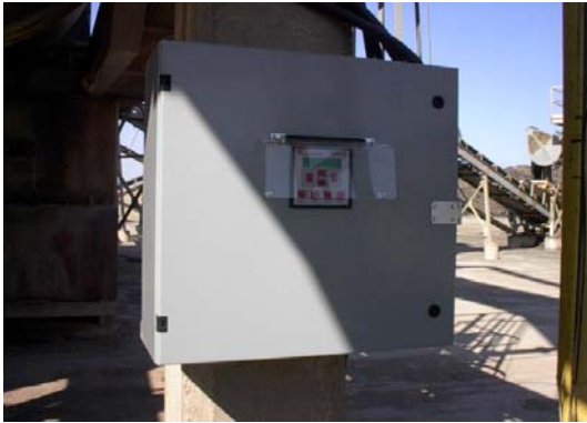
Front view of the main control panel (Fireye Nexus PPC-5000 ) for the Asphalt Kiln burner with the Fireye Nexus Display.
