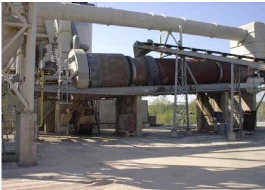
Side view of the Asphalt Kiln with the burner on the middle left.
